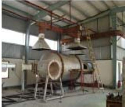
Lead Smelting Plant (Under Process)
