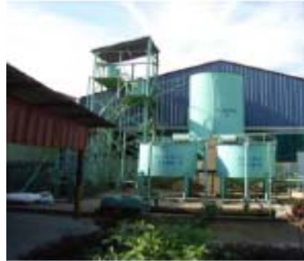
ETP for Battery Manufacturing
