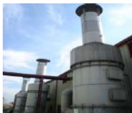
Acid fume removal scrubber (Formation unit)
