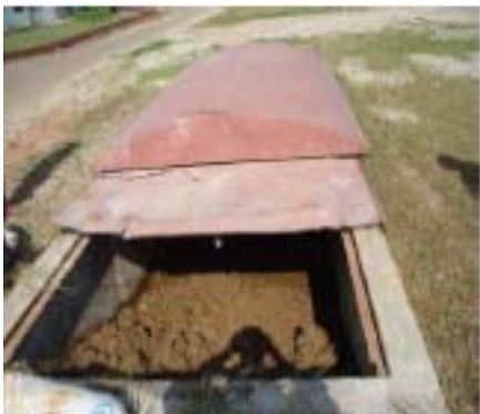
On-site sludge storage tank
